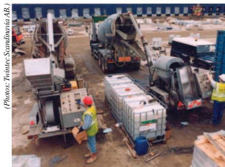
Figure 1: The most effective way of incorporating the steel fibres is with a pneumatic 'blast' machine.
