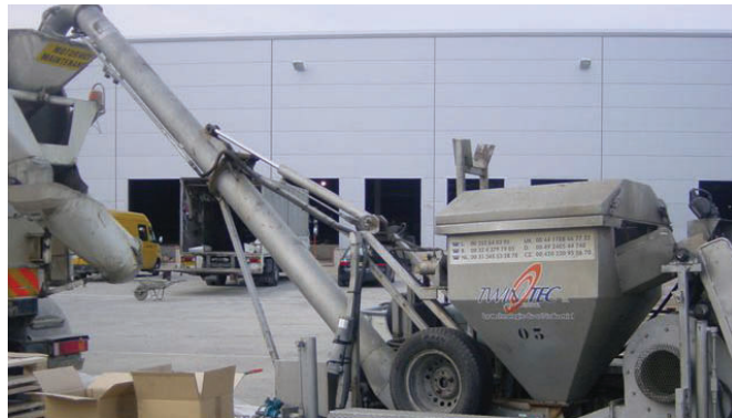
FLOORING WORK GETS UNDERWAY ON PART OF THE AL AZIZIA DC IN RIYADH.
